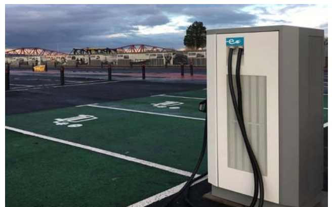
Electric Vehicle Bays at the Forth Road Bridge
